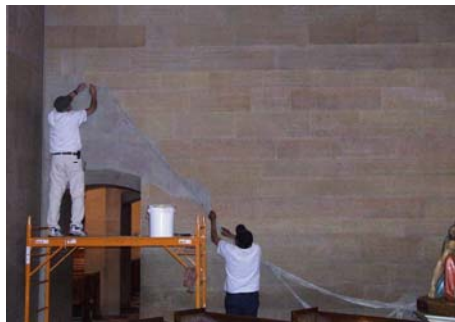
E. Removal of ABR ® Waterless Cleaning Poultrice in one piece from large wall section.
